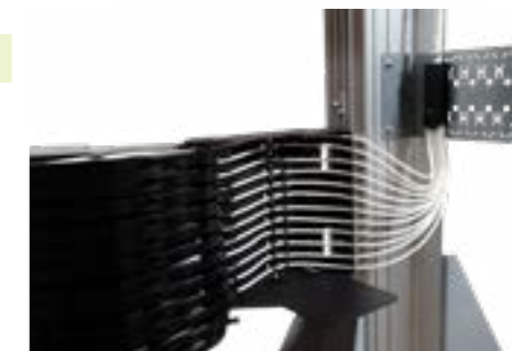
Management of protection tubes.
