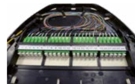
Connection example in an iTOM-V3 rack
